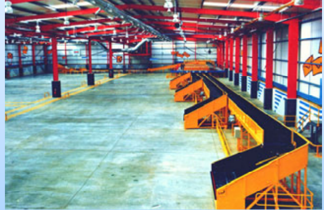
Belt conveyor system handling mail bags for sortation
